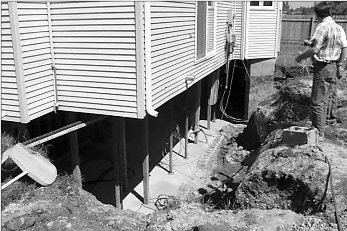
Figure 9 Failure of this unreinforced masonry basement during flooding in East Grand Forks, MN, in 1997 caused approximately $32,000 in damage.
